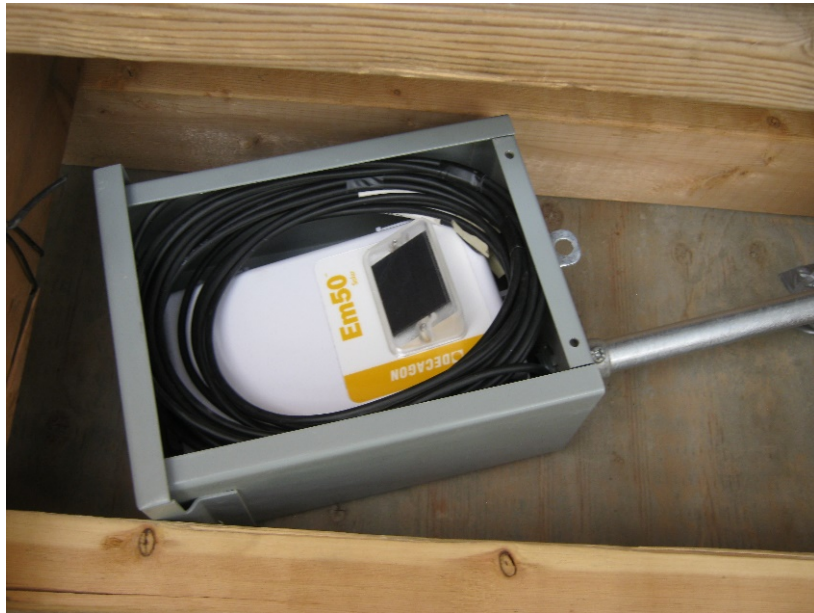
Figure 3-3: Data logger mounted inside a junction box.
