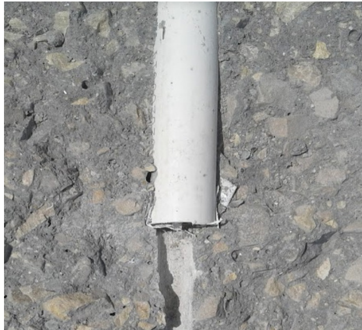
Figure 4-44: Shear Failure of the Concrete as Observed by a Smooth Surface Being Left on the Concrete
