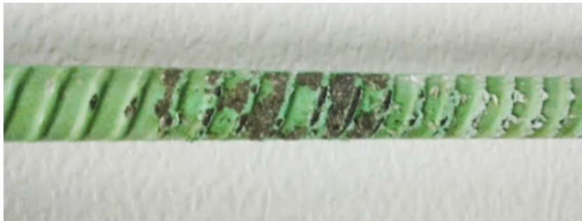
Figure 4-39: Rebar Surface Failure on Steel Epoxy Coated Rebar
