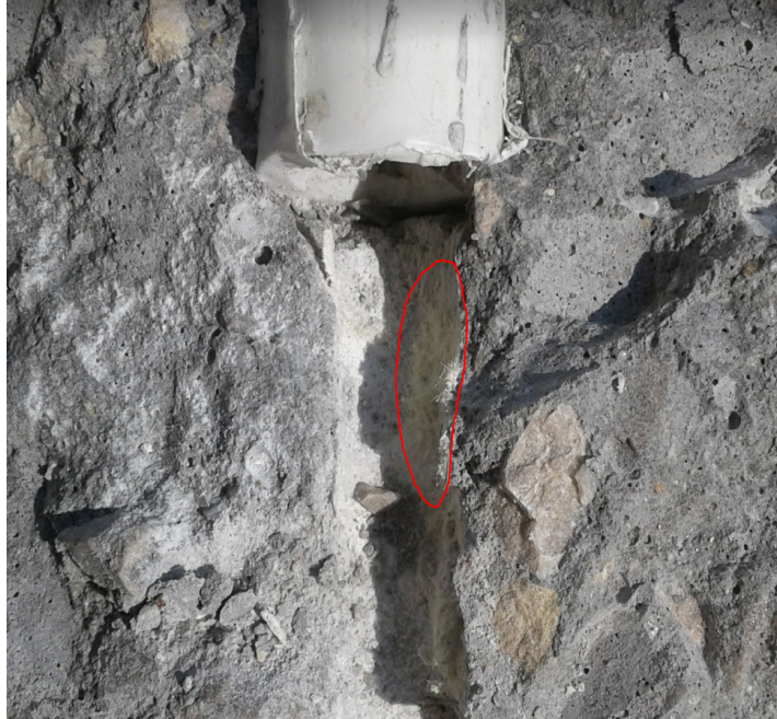
Figure 4-43: Rebar Coatings Left on the Concrete after Pull-Out
