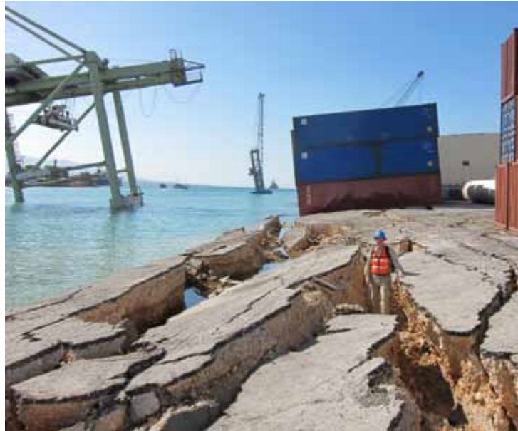
Figure 4-2: Example of lateral spread displacements causing fissures along a port in Haiti after the 2010 earthquake (after Eberhard et al. (2013)).
