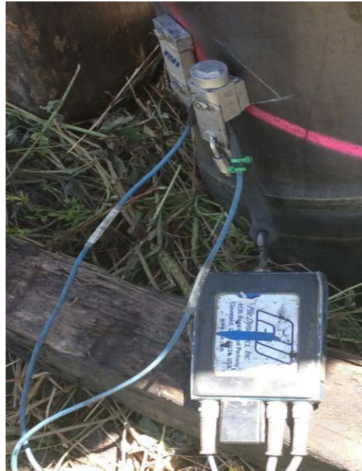
Figure 4.4-1 Accelerometer and strain gauges connected to the top of a pipe pile at the end of driving in connection with PDA measurements.
