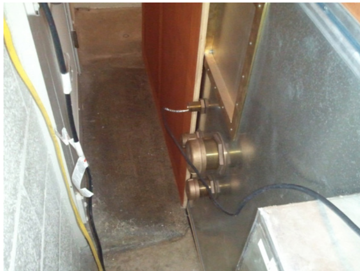
Figure 4-10. Outside view of coupling connections on BYU's Faraday cage.
