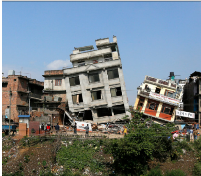
Figure 4-2: Buildings tipped over from differential settlement from the 2015 Kathmandu, Nepal earthquake (after Williams and Lopez, 2015).
