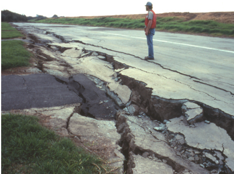
Figure 3-20: Lateral spreading from the 1989 Loma Prieta earthquake.
