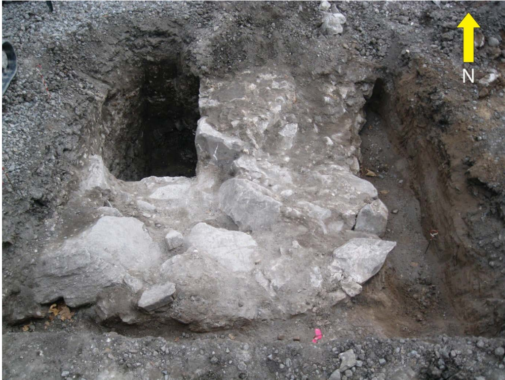
Figure 4.5. Photograph of initial test pit showing the southeast corner of the OPT foundation (image courtesy of OPA).
