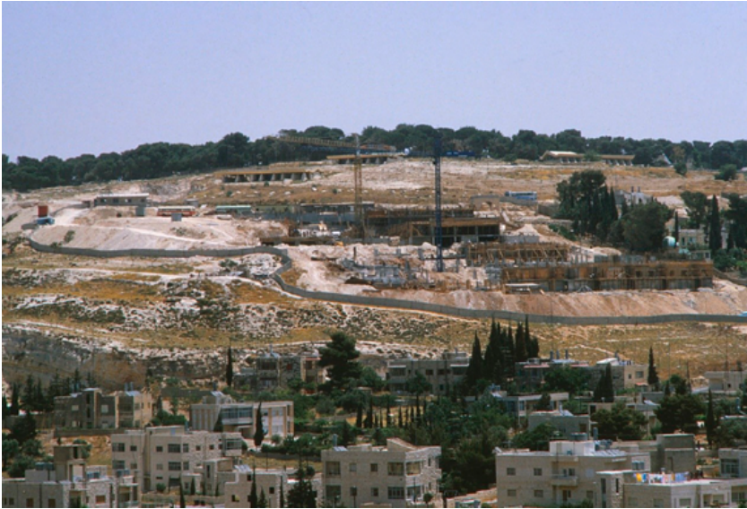
FIGURE 1. BYU Jerusalem Center under construction in June 1985. Photo courtesy Jeffrey R. Chadwick.
