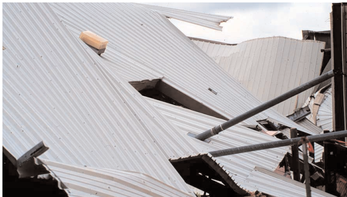
Fig. 2. The collapsed west end of the building, providing an access ramp to the roof.
