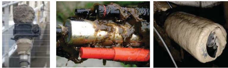
Figure 1. Examples of faulty sensors.
