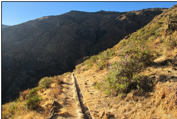
Figure 3.8. Cement canal with historic stone foundation visible on either side located above the village of Llancha between the sites of Huarmishcoto and Puquio Sangre. Photo looking northeast at the peak of Shaucañí.
