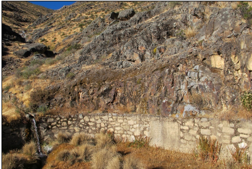
Figure 3.11. Large cement plaque on the wall of the reservoir at Puquio Sangre.
