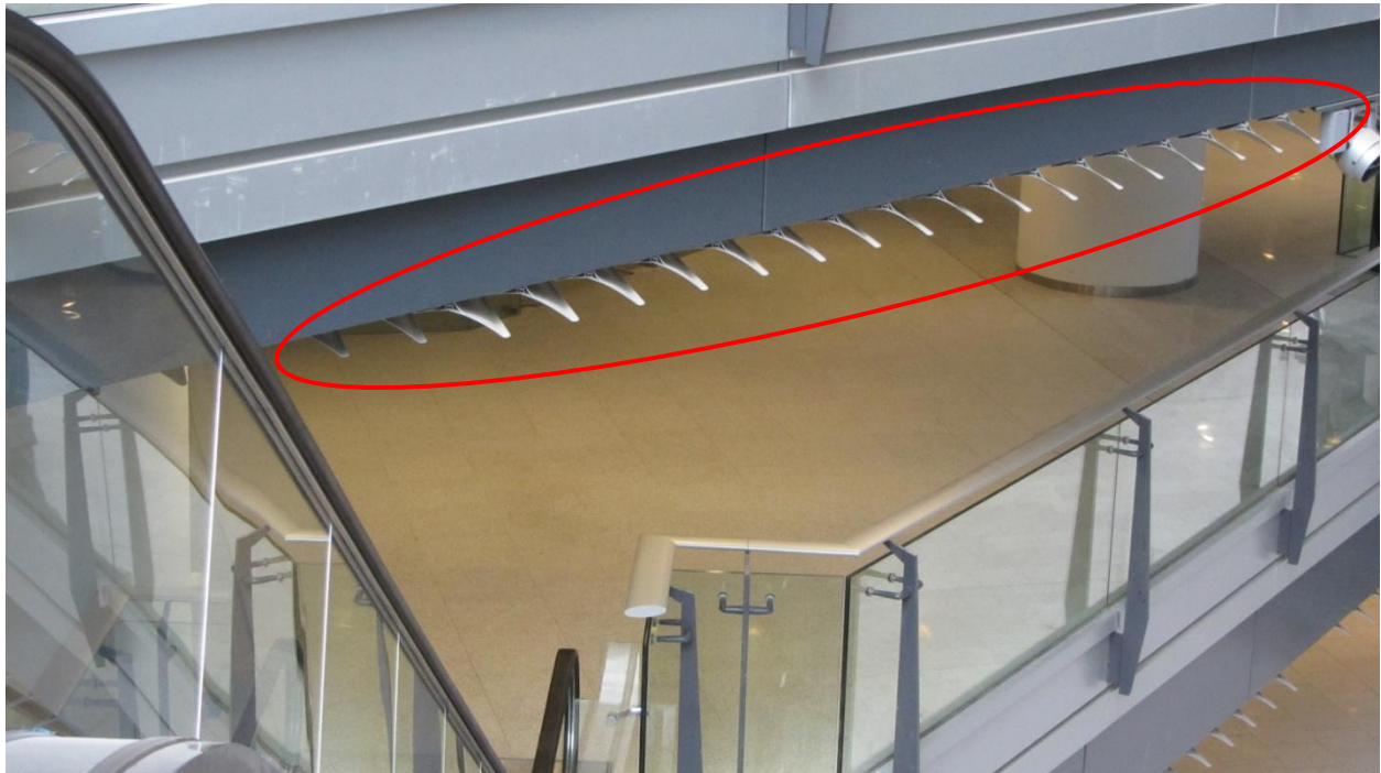
Figure 2-4 Hydronic cooling fins under balconies in the Parkview Green atrium
