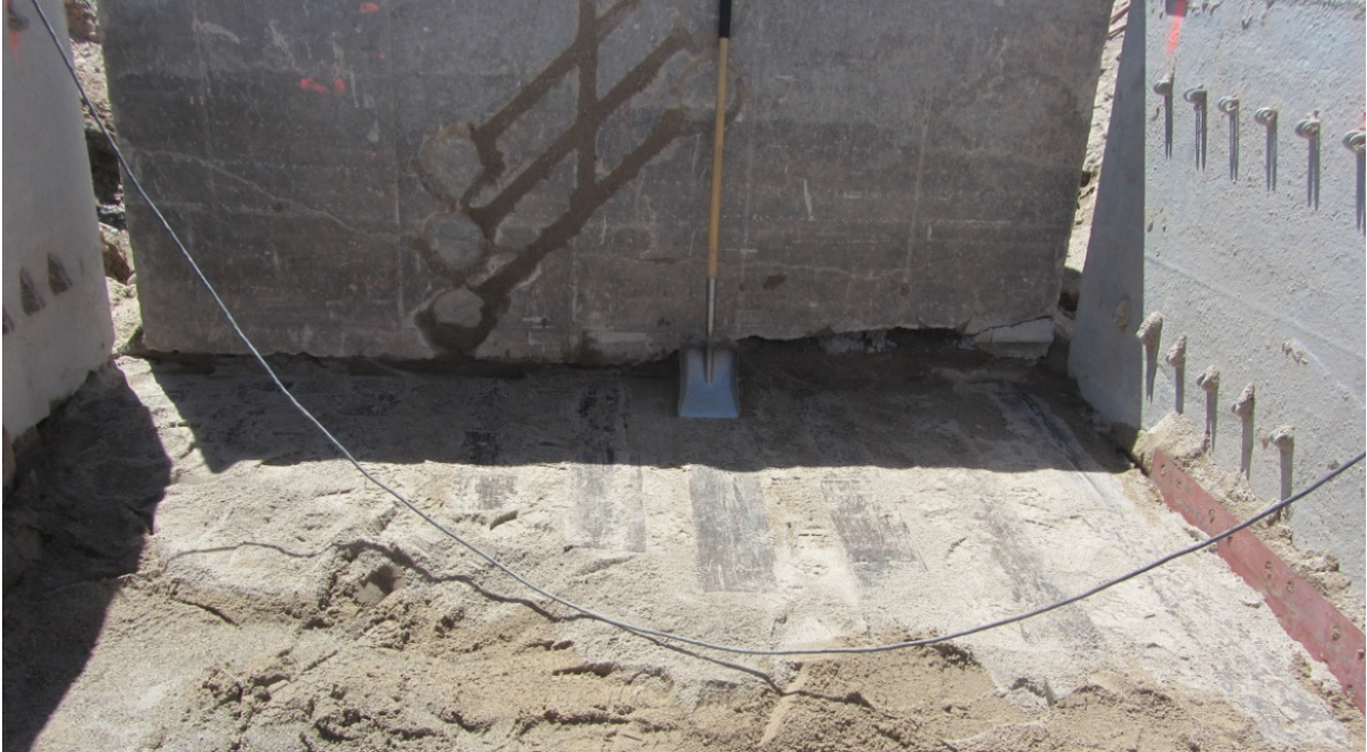
Figure 3-9: Railroad tie foundation for 15° and 30° wedges with sand compacted between ties (Marsh, 2013)
