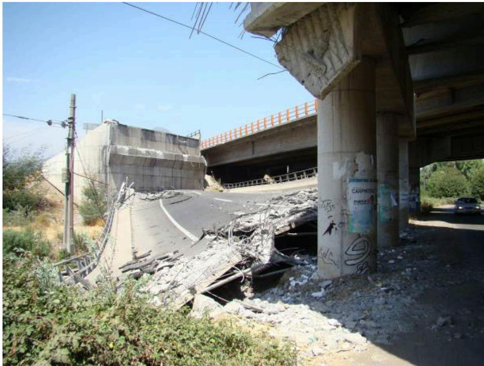
Figure 2-22: Collapse of skewed bridge deck adjacent to a functioning normal bridge. Chile Maule earthquake, 2010 (Unjohn, 2012)
