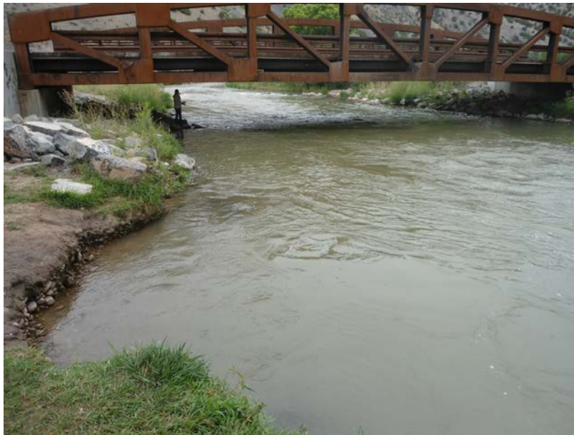
Figure 2-4: Abrupt Change from Riprap to Streambank, Causing Downstream Scour. Flow from Top to Bottom (picture taken by Evan Cope).
