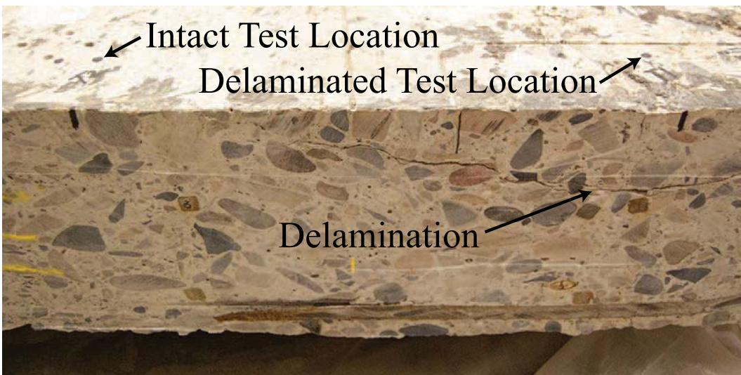
Figure 4.2: Intact and delaminated test locations on the concrete bridge deck sample.
