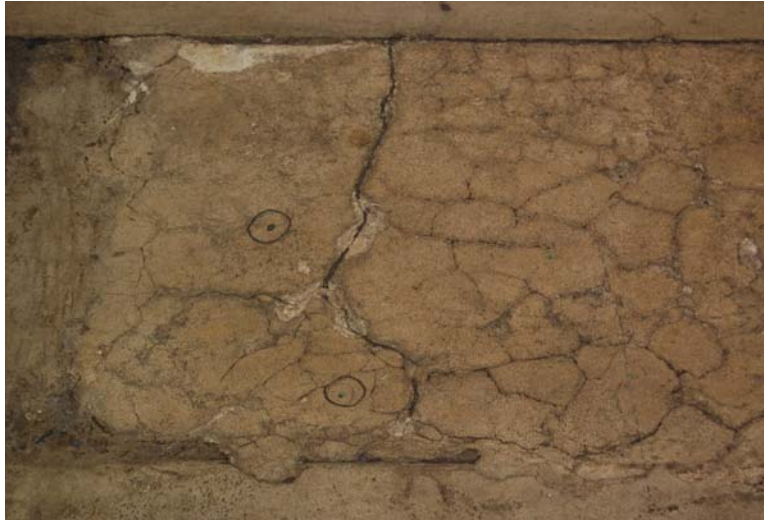
Figure 3.1: Photograph of the delaminated on-grade concrete floor in laboratory FB-110 (Harvey Fletcher Building, Brigham Young University campus).
