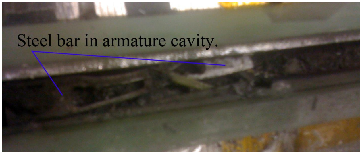
Figure 2-13: The remains of the steel bar backing used for one of the sensors.
