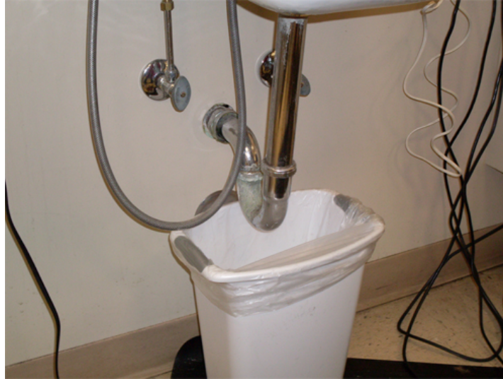
Figure 4-2: Photograph from Leaky Drain Problem-Finding Item
