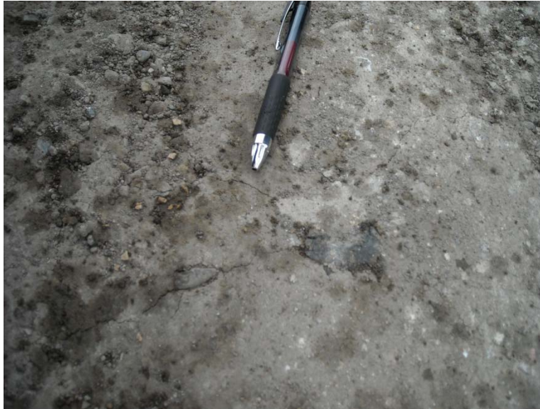
Figure 4-24: Fine cracks in CTB surface after microcracking.
