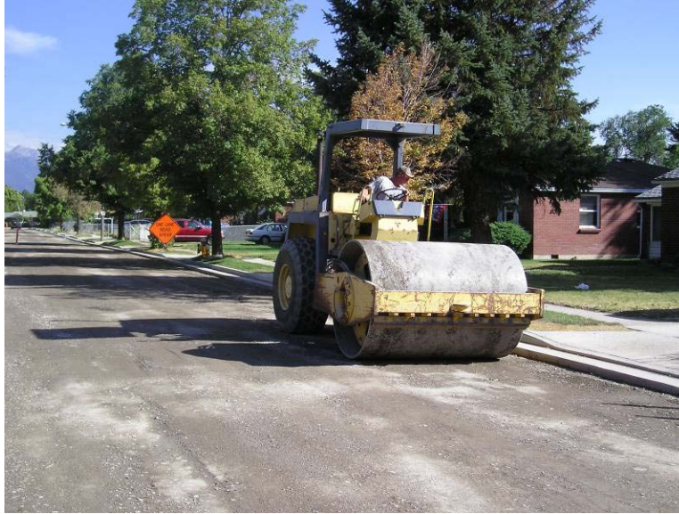
Figure 2-4: Microcracking using a vibratory roller.
