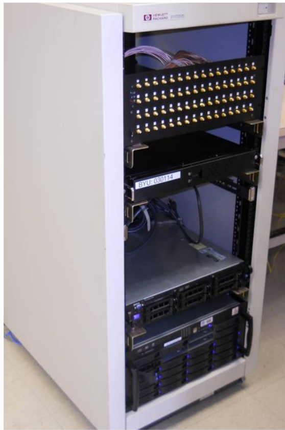
Figure 6.4: Equipment rack configuration with ROACH and 64 RF input connections for the x64adc (top), a second ROACH which will perform beamforming operations (middle) and host computers and data file server (bottom).
