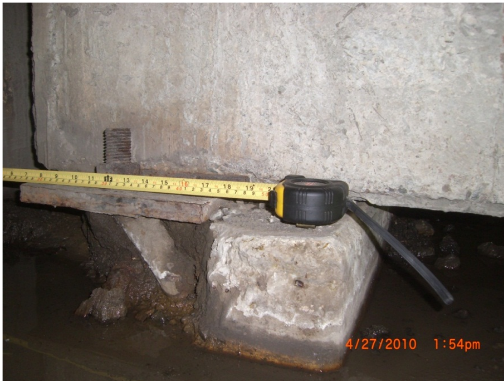
Figure 8-4: Displacement at the Base of the Bridge Girders
