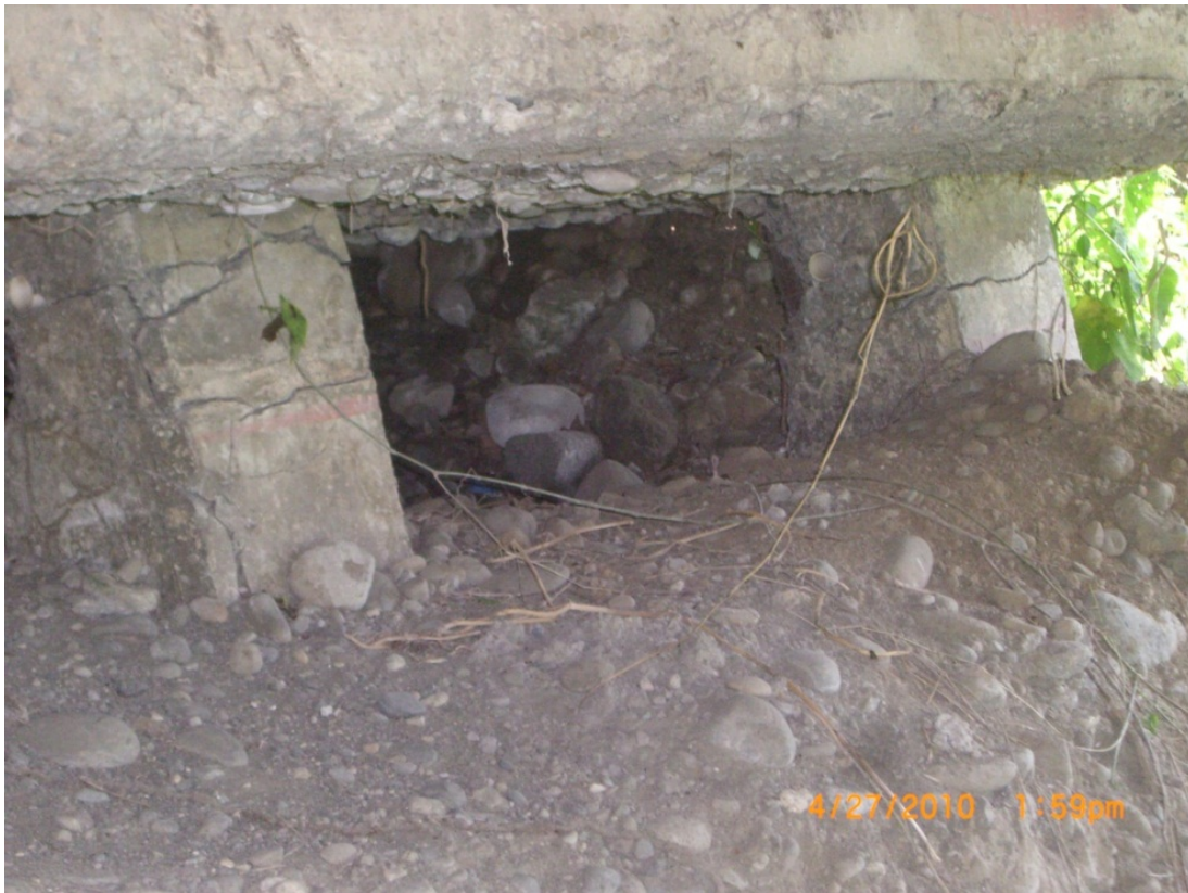
Figure 8-5: Pile Cracking Observed at the East Abutment of the Rio Cuba Bridge
