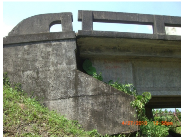
Figure 8-2: Rotation of the East Abutment at the Rio Cuba Bridge
