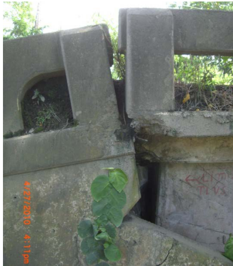
Figure 9-2: Rotation of the Pile Cap at the East Abutment of the Rio Blanco Bridge
