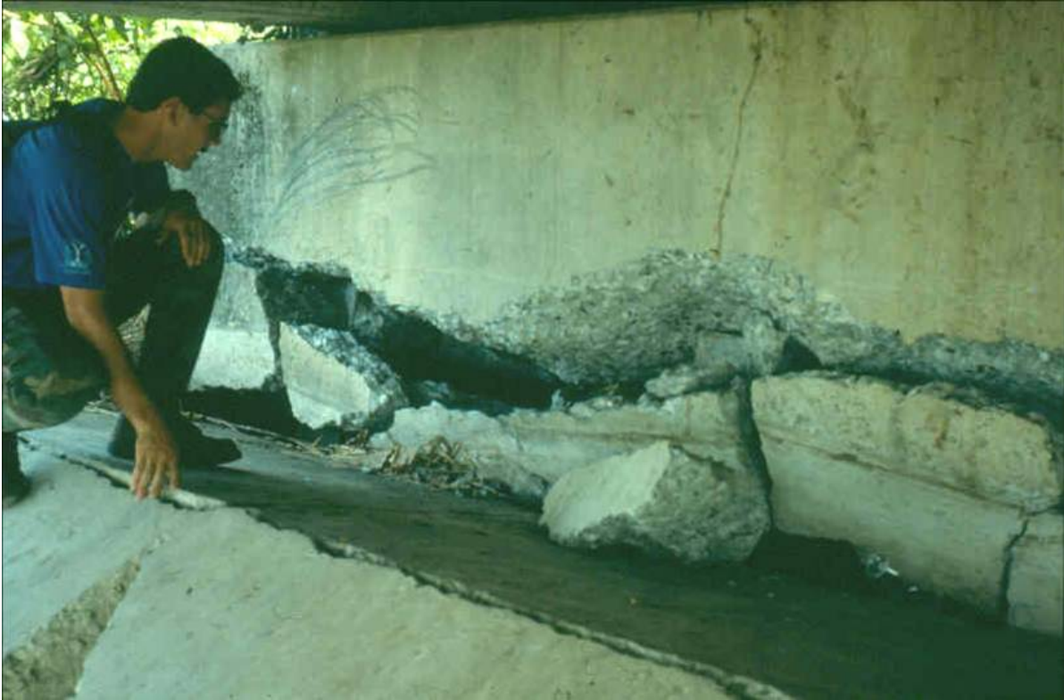
Figure 10-2: Rotated Pile Cap at the South Abutment of the Rio Bananito Highway Bridge
