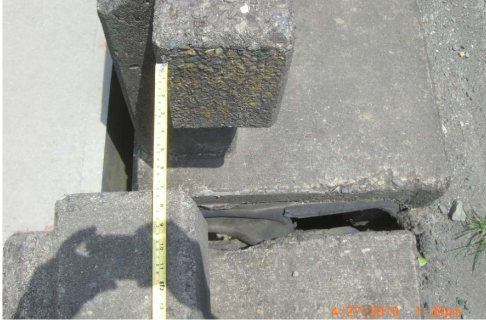
Figure 8-3: Transverse Displacements at the Bridge Deck at the Rio Cuba Bridge
