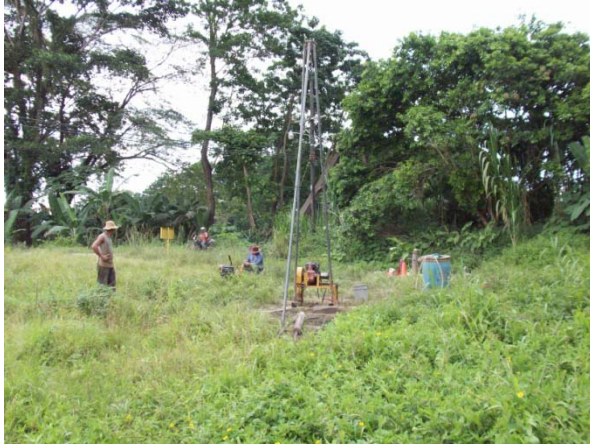
Photo 5: View of the site of borehole P-1 at the Rio Bananito Railroad Bridge. The borehole is on the left margin of the river.
