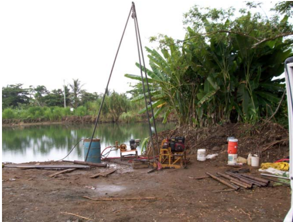
Photo 3: View of the site of borehole P-1 at the Río Bananito Highway Bridge. The borehole is on the right margin of the river.
