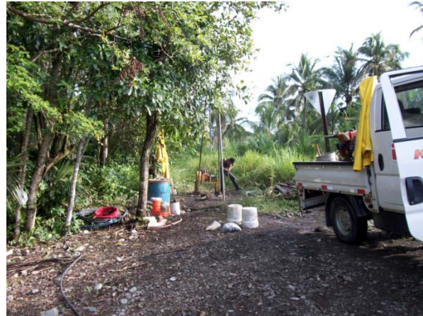
Photo 4: View of the site of borehole P-2 at the Río Bananito Highway Bridge.
