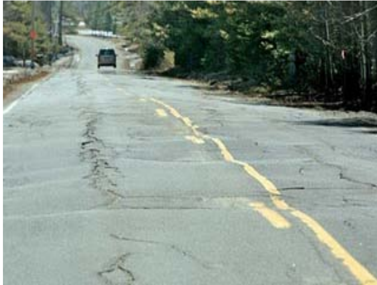
Figure 2.3: Pavement damage due to frost heave (37).
