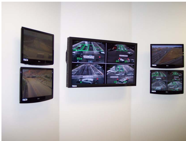
Figure 3-5: BYU Transportation Lab monitors
