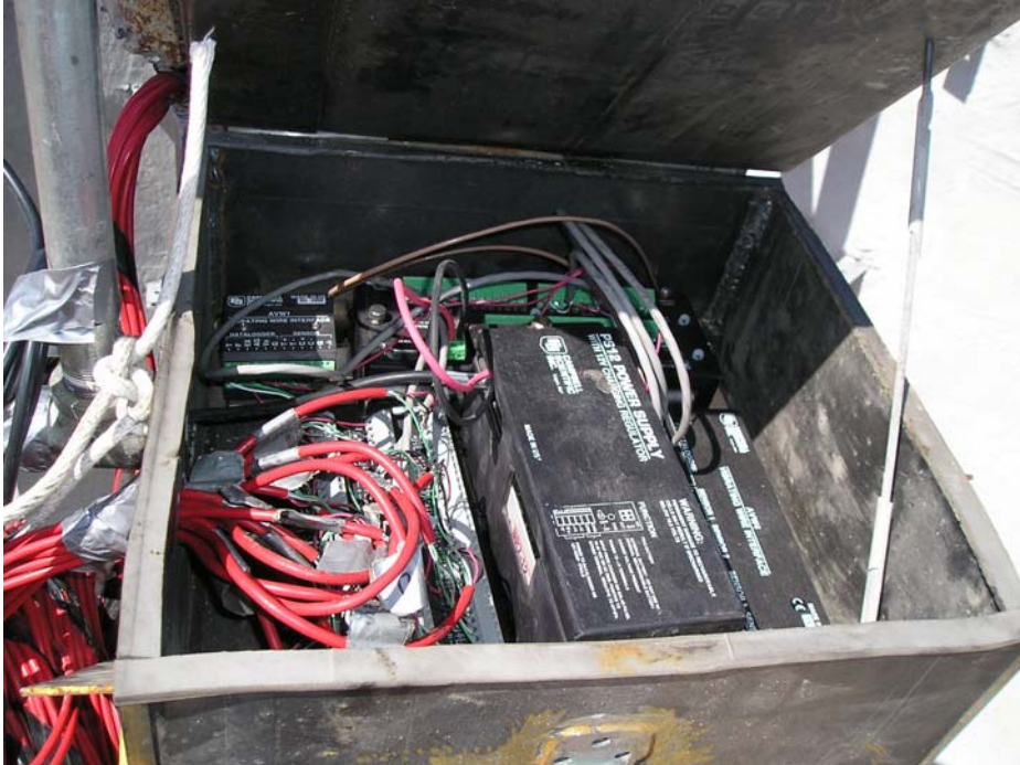
Figure 4-10 Data Logger with other Components and Wires Attached
