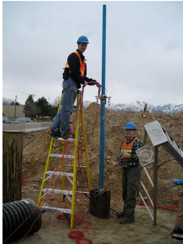
Figure 4-8 Installing Pipe Sections One at a Time at Redwood Road and SR-201 (author photo)
