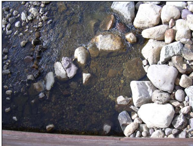
Figure 4-22. Bendway Weir on the North Fork Provo River After Runoff.
