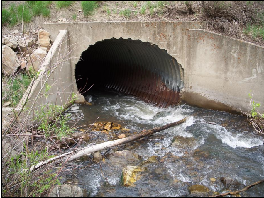
Figure 5-42: Hydraulic Jump Just Upstream of Inlet
