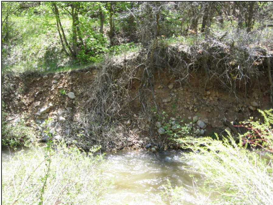
Figure 5-26: Stream Bank Erosion
