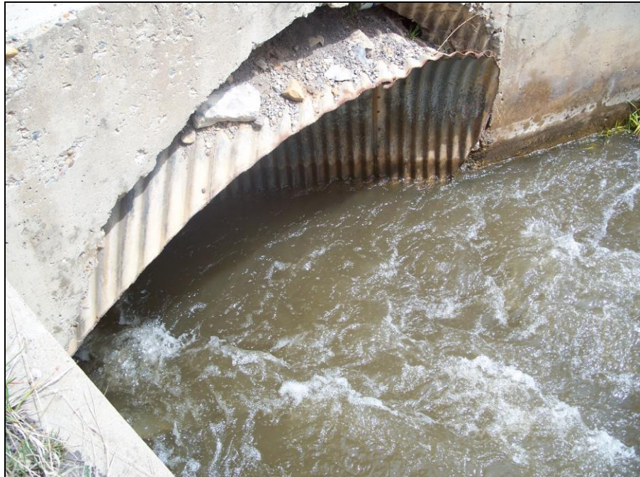
Figure 5-27: Culvert Separating from Headwall
