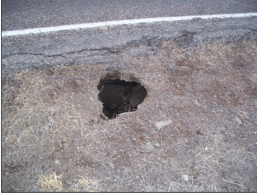
Figure 5-28: Possible Road-Side Erosion Associated with Figure 5-27
