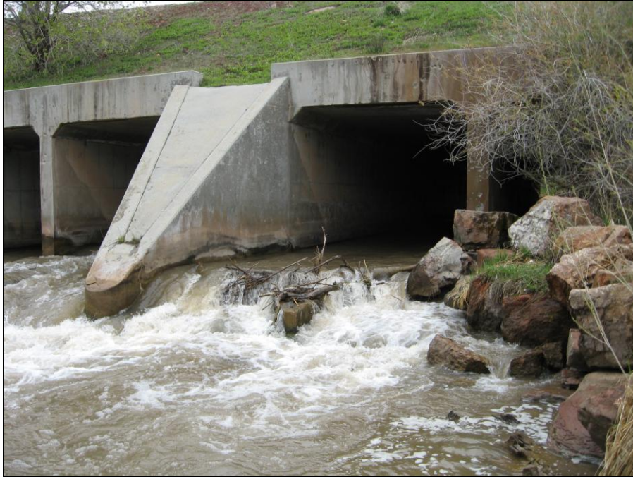
Figure 5-17: Debris Pile at Culvert Outlet
