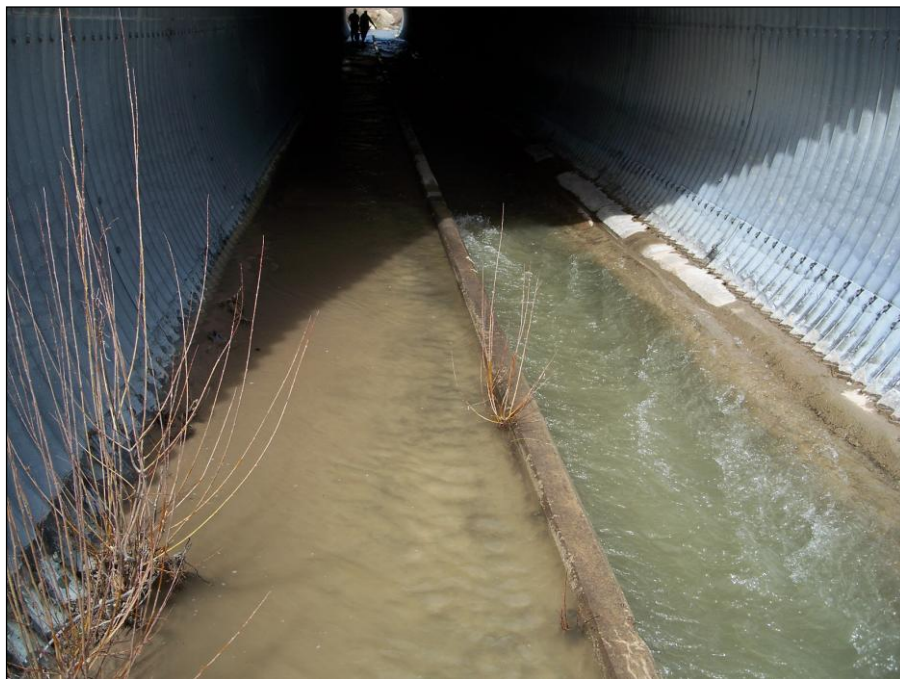
Figure 5-10: Wildlife Trail in Culvert
