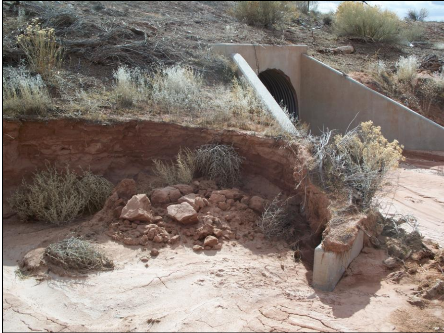
Figure 5-25: Erosion Behind Wingwall
