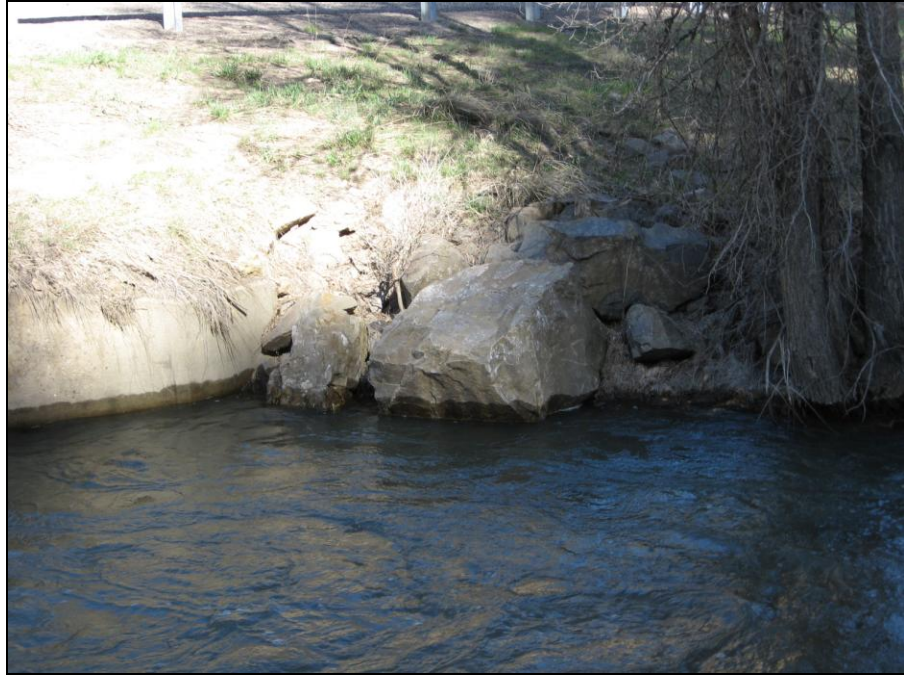
Figure 5-21: Riprap at Toe of Outlet Wingwall
