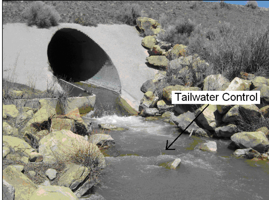
Figure 5-5: Outlet and Tailwater Control Photo
