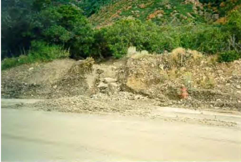
Figure 11: Preston Canyon Drive where the debris flow crossed Bald Mountain Drive, photograph taken facing east. (September 18, 2002)
