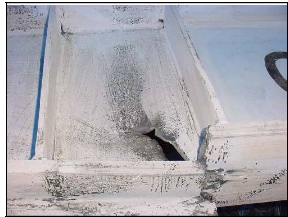
(b) Fracture of Beam Flange
