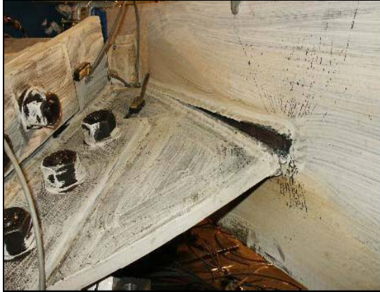
(a) Fracture of Gusset-to-Beam Weld
