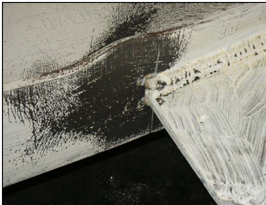
(c) Fracture of Beam
