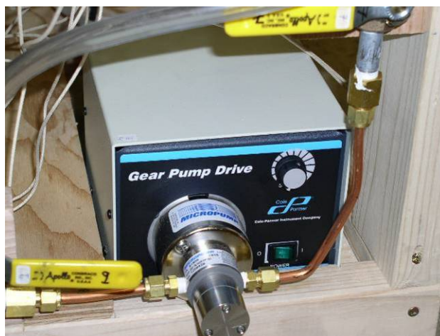
Figure 21. Liquid Pump, P-101.
