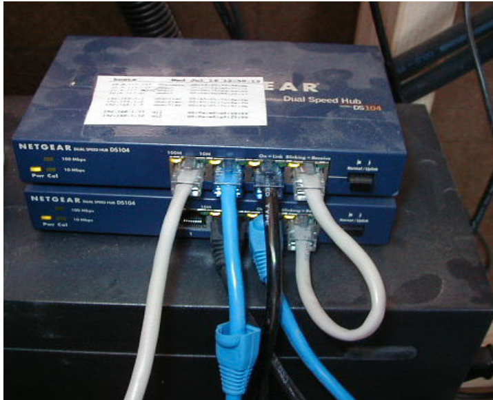
Figure 31: Network communication via standard Ethernet components
