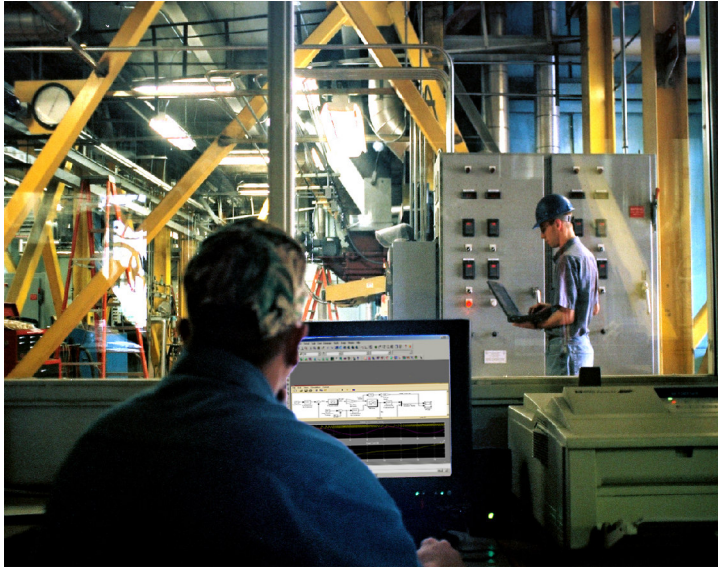
Figure 6: BYU heating plant
