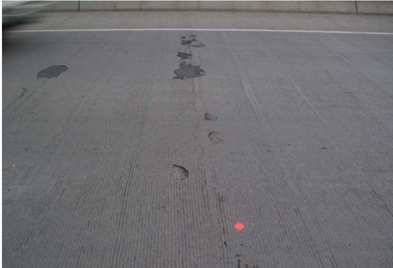
FIGURE 4.37 Transverse cracking and potholes on bridge C-635.
