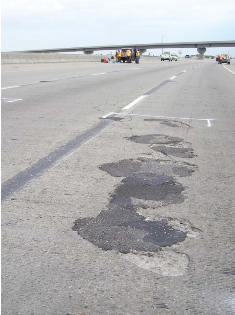
FIGURE 4.40 Localized spalling of concrete on bridge C-704.
