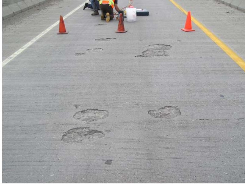
FIGURE 4.41 Transverse cracking and potholes on bridge C-702.
