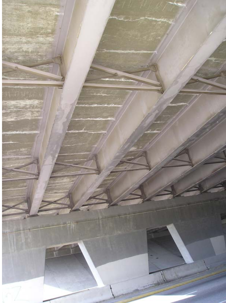
FIGURE 4.39 Transverse cracking with efflorescence on bridge C-693.
