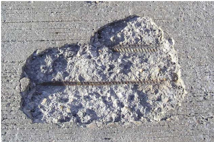
FIGURE 4.38 Exposed reinforcement in pothole on bridge C-460.
