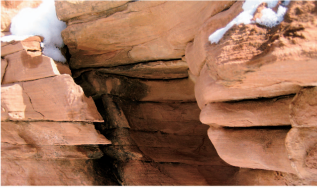
Fig. 1. Spheroidal weathering in soft sandstone. Spheroidal weathering will eventually reduce the sharp edges on the left to the rounded edges seen on the right.
